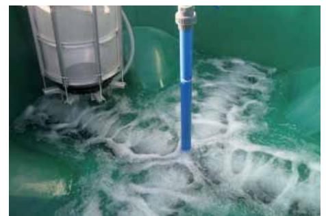
The bubbling pipes in the tanks. The stainless steel sieve aerating the compost is also visible.
